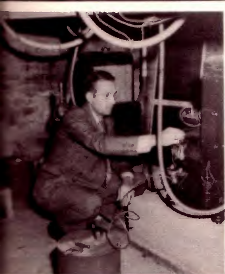
The KFJZ Emergency Power Plant which Ed Starnes is adjusting is put into operation to continue normal service for KFJZ and TSN in the event Fort Worth power should be interrupted.
