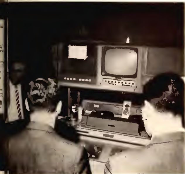
Other before lunch meetings included a tour of the station's generous facilities. In this instance, Charles King, WRGB manager of production, shows rep group the control room video tape unit
