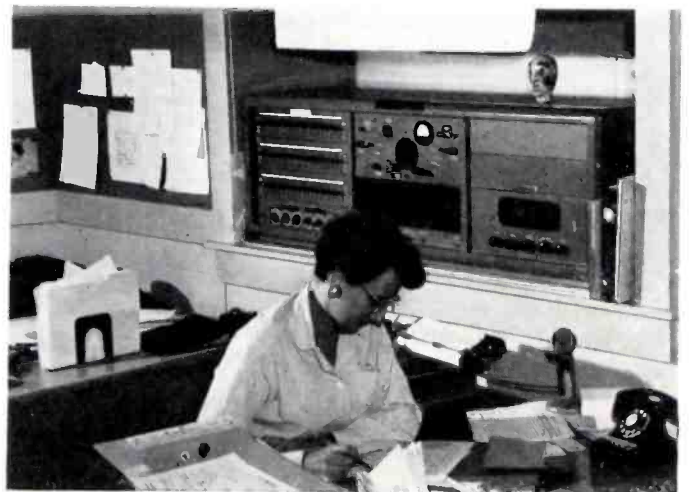
AN IMPORTANT PART of the city wired for sound is its school system. Kunze was responsible for the installation of this modern school console sound system in Racine's Washington Jr. High School.
