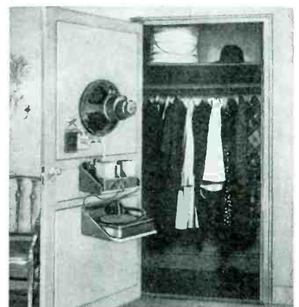
Fig. 2c. Duplex speaker and associated hi-fi units installed on back of a closet door. (Courtesy Altec Lansing)
