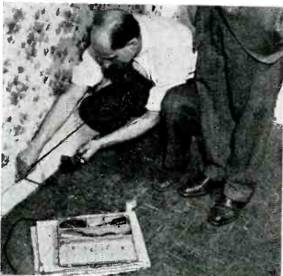
Fig. 11. Tacking transmission line to baseboard. Note that the tool box rests on a protective cloth. Incidentally, small tack hammer is preferred over the heavy work hammer shown in this illustration.
