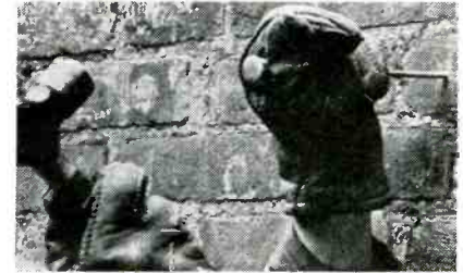
Fig. 2. Making a hole in a brick wall with a rawl tool to facilitate drilling larger hole with an electric or star drill. Note the use of gloves to protect the hands and also keep them clean.
