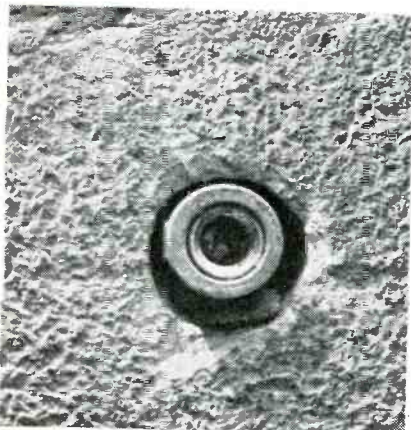
Fig. 4 (above). A lead expansion fitting inserted into hole made by a star drill. The surface flaking around hole is common when the star drill is used to make holes in aged brick.
