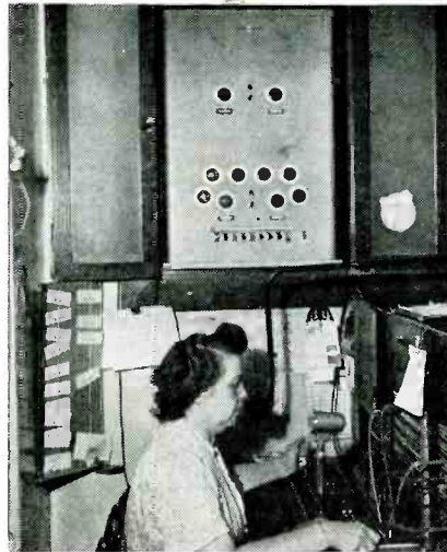
Fig. 1. Alarm and speaker setup at telephone switchboard in apartment-hotel.
