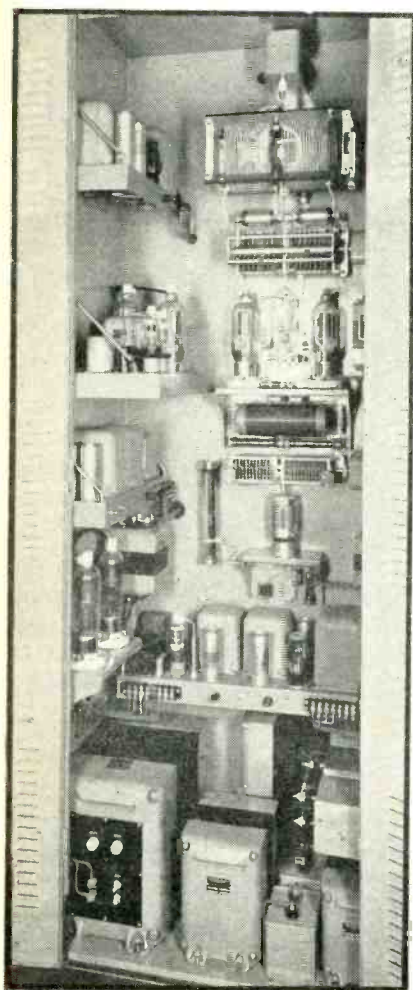
Interior of 250-watt AM transmitter. Silent natural draft ventilation is used
