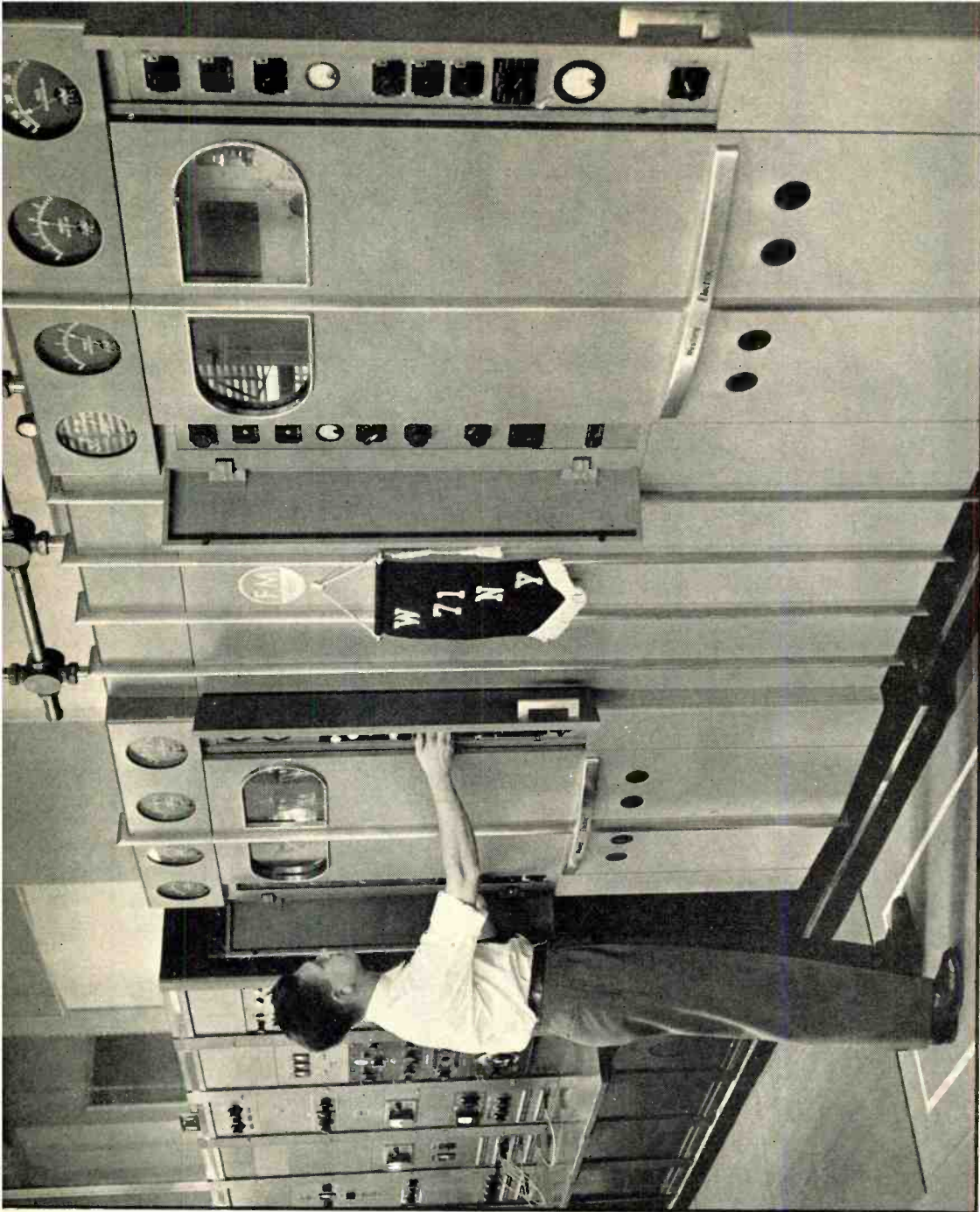
The new 10,000-watt transmitter of W71NY, frequency modulation station of WOR, New York, which was dedicated on Sunday, Nov. 30th. The transmitting plant is located at 444 Madison Ave., New York City.
