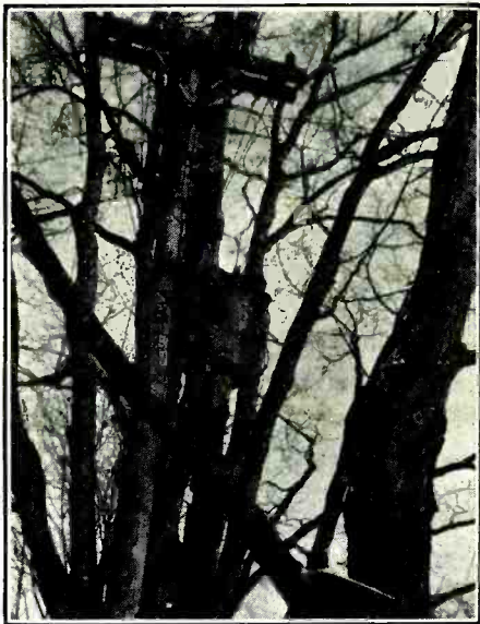
FIGURE 1. Transformer installed among trees. Many grounds.
