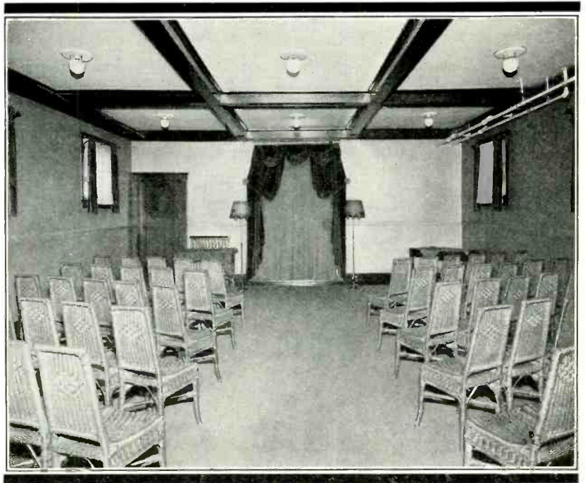
A unique sound equipment installation in funeral parlor of Ritter & Son, Milwaukee, Wisconsin. WRIGHT-DE COSTER SPEAKER is mounted in back of drapes in center, and music is furnished continuously by phonograph with automatic record changer. As a result, much of the gloom is dispelled.
