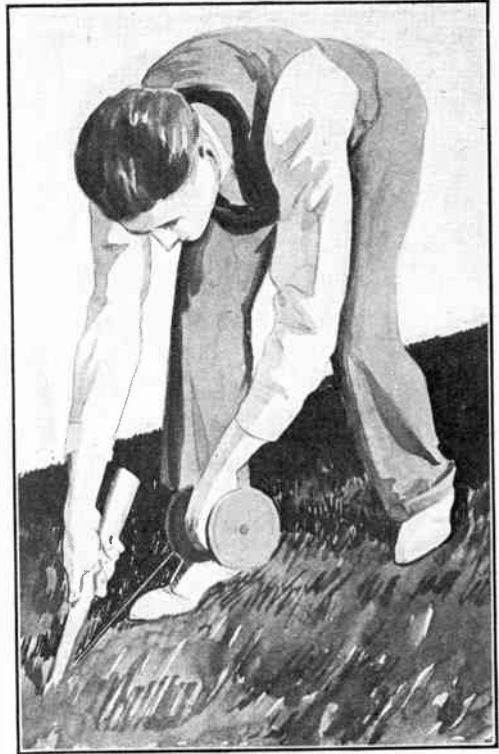
A buried ground wire is the basis of a new noise-reducing system. To lay the wire the author had wire spool in one hand and guided the wire in grooved plywood to force the wire into the ground. The method supplanted axe for handplow (above).
