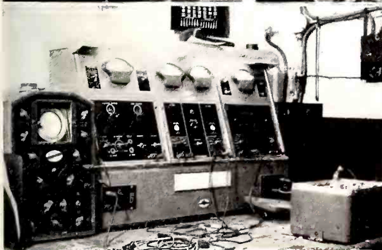
6. Set operates on test bench long enough to show up any drift, or suspected part failure. Preliminary alignment is made on the bench, but some sets require additional adjustment of RF padders after set has been put into the car.
