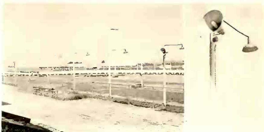
Roosevelt Raceway's 25-watt University Lab speakers, at Westbury, L. I. Sound installation man was Walter Bickmeyer, 116 Main St., Hempstead, N. Y. Speakers are used for announcing to race crowds.
