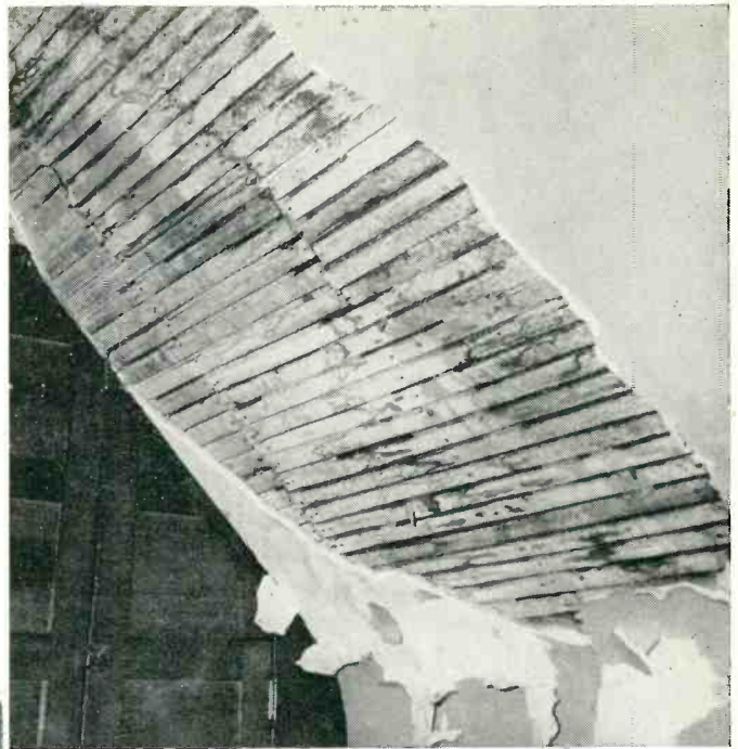
Fig. 4 (top). The shock was so violent that the ceiling plaster in an adjacent room was damaged over a wide area.
