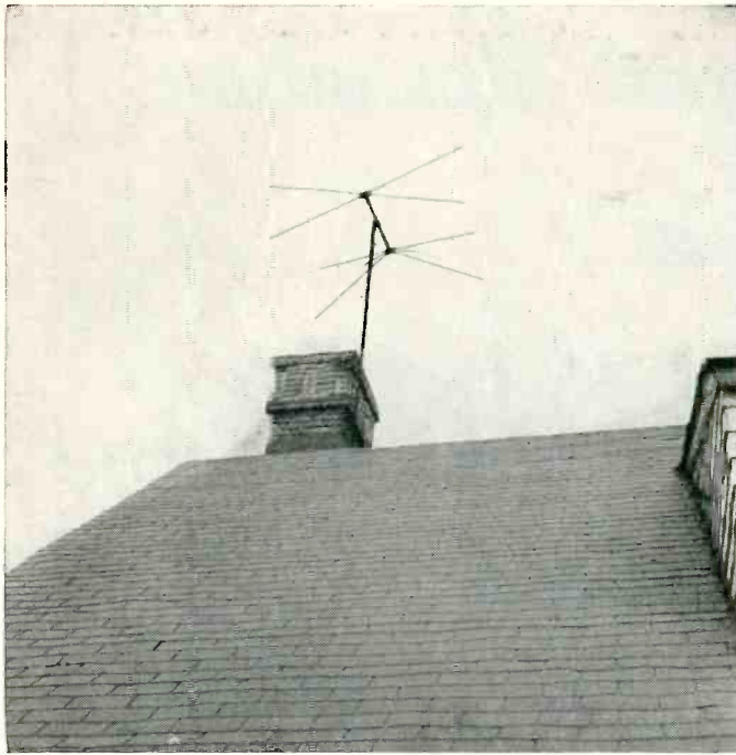
Fig. 1 (top). This is the TV antenna that was struck by lightning. Notice the absence of the downlead which was ripped off by the stroke.
