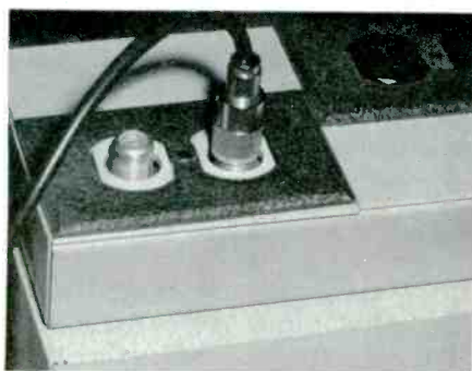
TV signal tapoff shown here supply signals for two demonstrator TV receivers. Note that it is located in a relatively "hidden" area and is positioned adjacent to a dual-receptacle power outlet. (Courtesy of Blonder - Tongue.)
