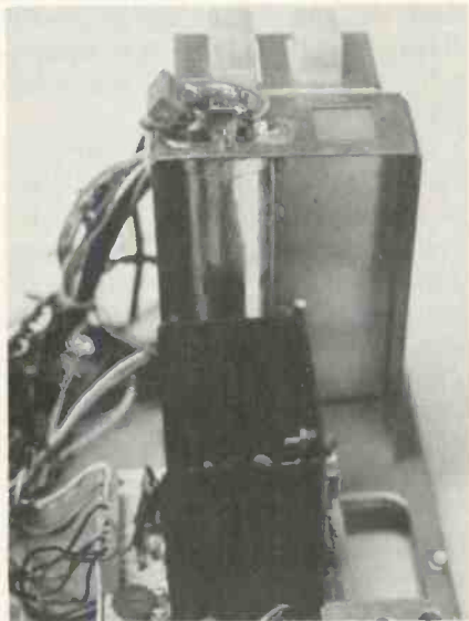
The filter capacitors are wired at the top to simplify removal, if required. Also shown are two of the wire harness plug-in connectors.
