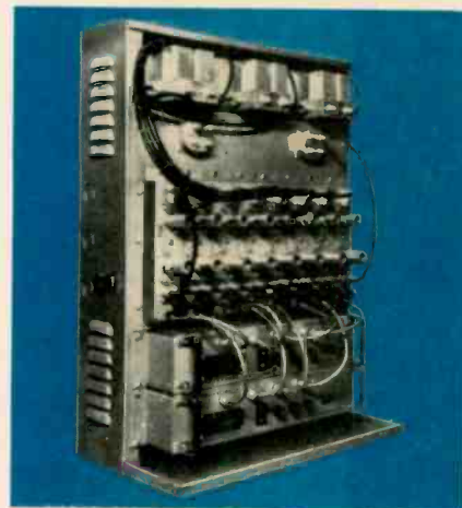
Single channel amplifier strips mounted in cabinet.
