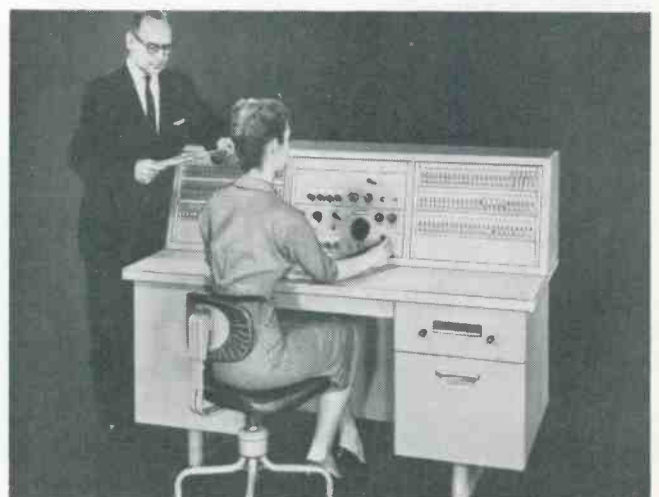
Multi-channel school console incorporates intercom and program distribution to all classrooms from microphone, tuner and phono.
