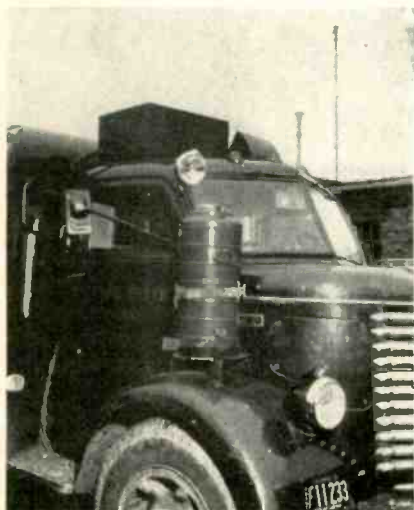
Mobile units used by utility companies are housed in heavy steel all-weather boxes and placed to take up minimum usable truck space. Here complete unit is in housing atop truck cab, with battery and control cables fed through flexible metal conduit to truck cab.
