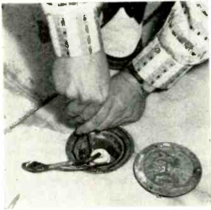
Fig. 3—Speaker leads and amplifier leads are connected to a flush-mounted deckbox.
