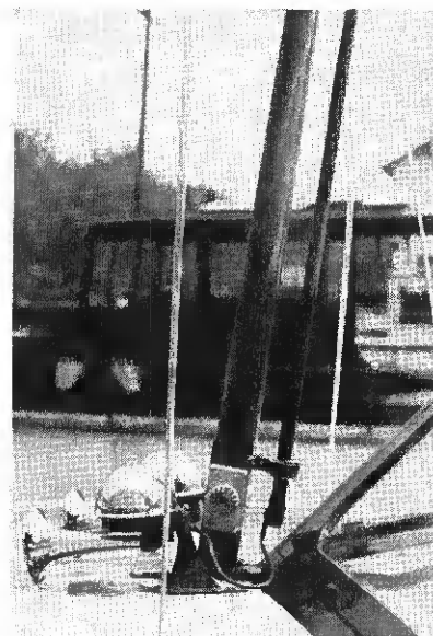
Fig. 1—Neat antenna installation on a small cruiser. Antenna is mounted along mast on screw eye insulators. Lead-in insulator can be seen under horns
