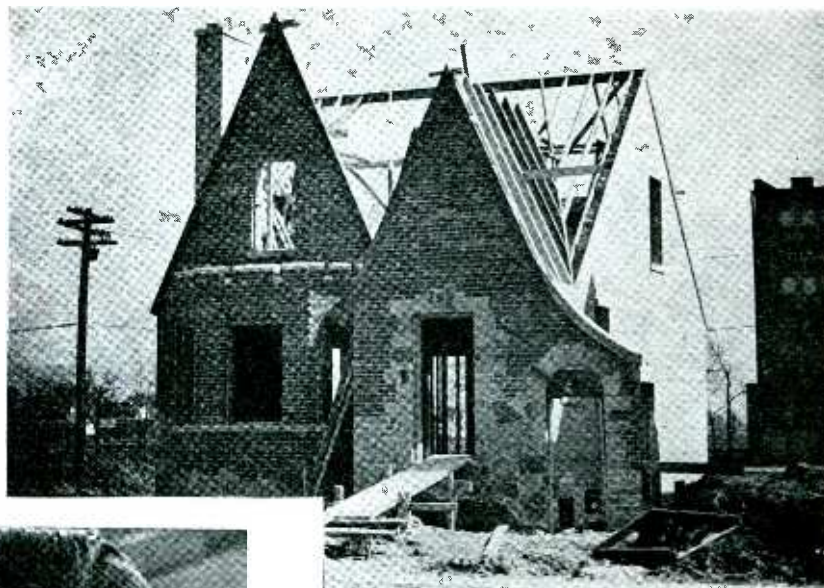
THIS IS THE TIME—Selling is most effective when exterior walls are up but before interior trim begins
