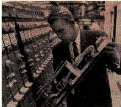
Bernie checks a unit in one of the operating consoles.
