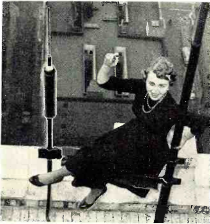
The mobile radio antenna installed 435 ft. above the street at Pacific Telephone and Telegraph's main building in San Francisco. Anne Flick doesn't mind the "long drop."
