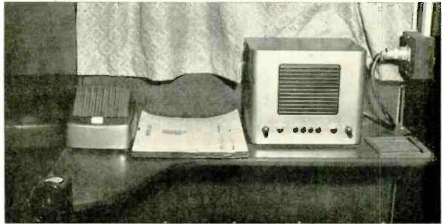
Typical "booth" or control point for one of the FM transmitters in the Center.
