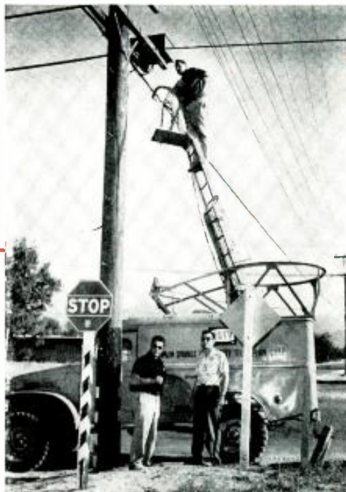
Service technician on a ladder truck used for repairing and maintaining community TV systems. The technician is checking a pole-mounted amplifier.
