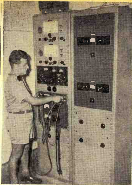
Close-up of main patch panel and compression amplifier. Capt. Panoff is shown setting up a radio circuit.
