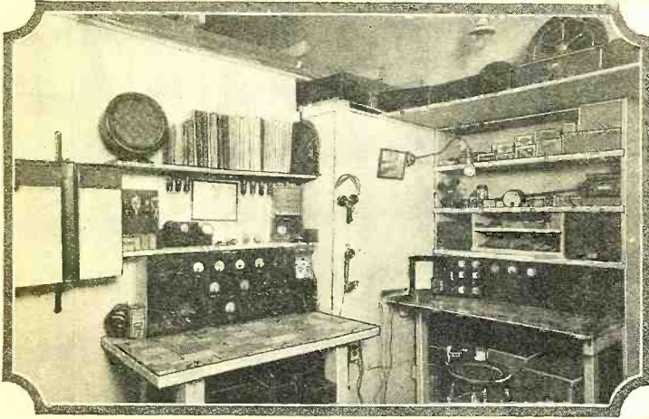
The picture above shows the service equipment of the Weslaco Electric Co., Inc., Rio Grande Valley, Texas. The equipment was built by G. C. McRoberts, a graduate of the Air Corps Technical School. Precision meters are employed exclusively in the permanent test panel and portable testers. A portable diagnetometer is used for outside servicing
