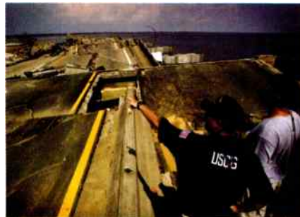
Jim Ward, left, of the Coast Guard, and Charles Berry examine the damage caused by Hurricane Katrina to a highway along the Casino Strip in Biloxi, MS, Wednesday, Aug. 31, 2005. (AP Photo/The Dallas Morning News, Barbara Davidson)
