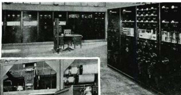
Transmitting room, Station WHAM. 5-kw. transmitter in the right foreground. —Courtesy, Western Electric Co.
