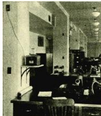
The photoelectric lighting control relay installed in an office for turning the artificial lights on and off without human supervision.
