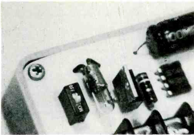
THE SMALL PILOT LAMP and the printed-circuit switch form a test circuit that permits the system to be tested without sounding the alarm bell. They can be eliminated if you want to cut costs.
