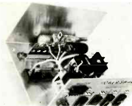
FIG. 3—THIS PARTICULAR VERSION of power switcher did not require 3-wire line cord, but yours probably will. Make sure that the ground wire makes good contact with case.
