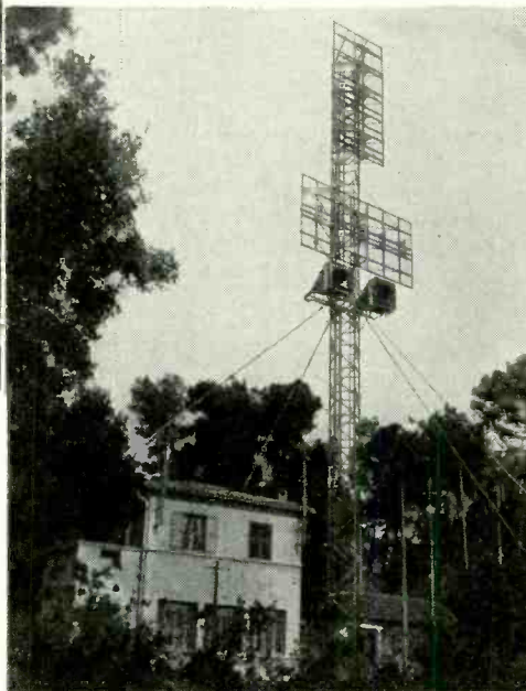
The microwave installation at Grasse on French mainland.
