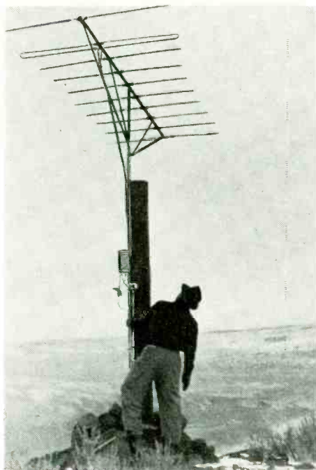
This unlicensed booster serves Bridgeport, Wash. Note complete transmitter on pole.
