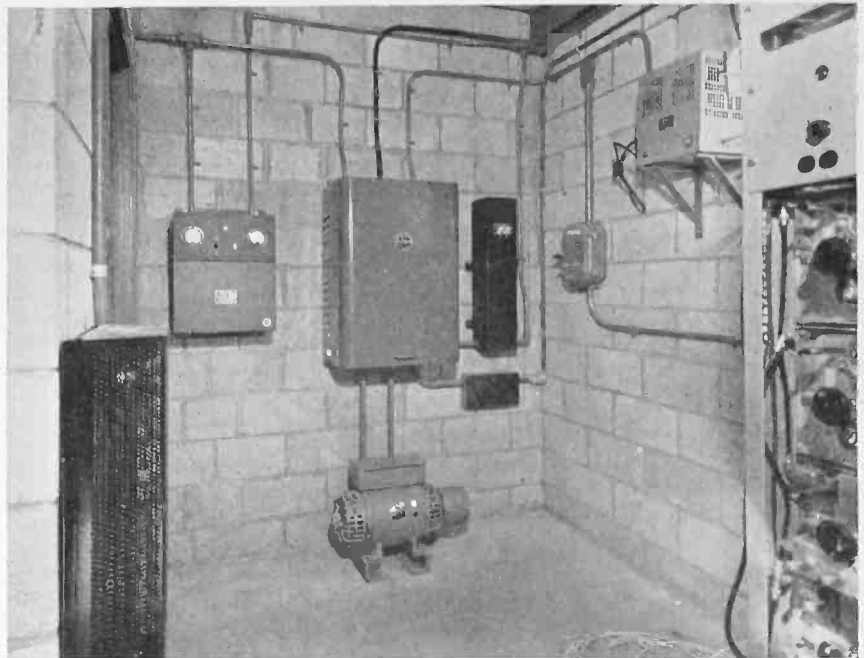
Fig. 1. Automatic battery charger, voltage regulating unit, and control unit for switching in emergency power when needed at the relay station.
