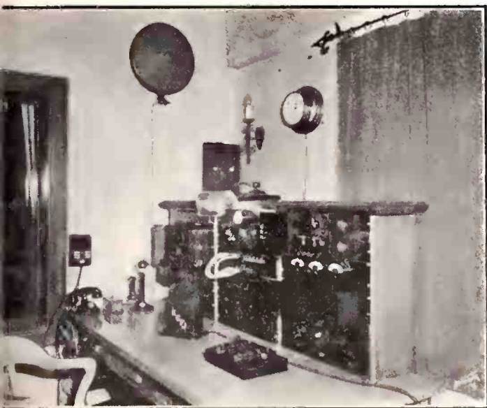
CONTROL ROOM—MODERN W. E. EQUIPMENT
