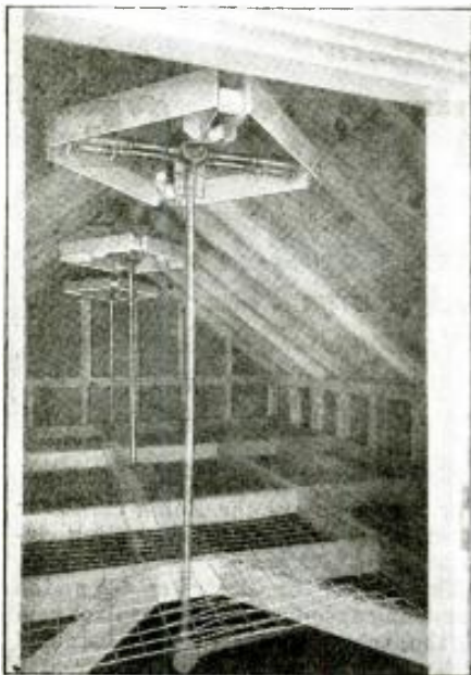
Here is shown the entirely new and unique 3-unit antenna installation for the runway localizer transmitters, of the new instrument-landing system, which radiates a horizontally-polarized "left-right" beam.
