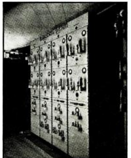
A portion of the amplifying equipment used in the super-power, 3-dimension sound system at the Lagoon of Nations, New York World's Fair, 1939. Frequency range: 28 to 11,000 cycles!
