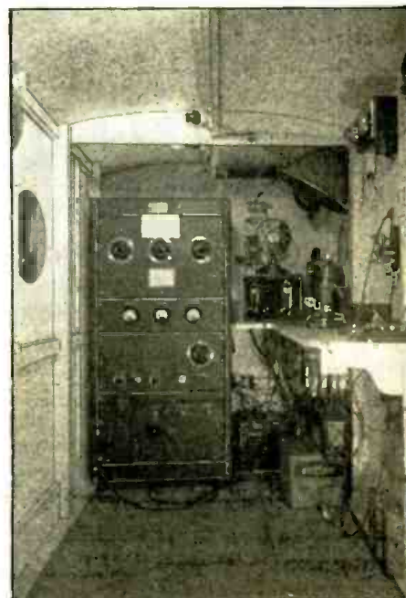
The radio, and line-telephone and -telegraph equipment are powered by optional generator or storage battery.
