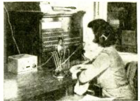
Practising what it preaches: the telephone switchboard at the "Wholesale Radio" office, showing the "mike" directly at the operator's elbow.
