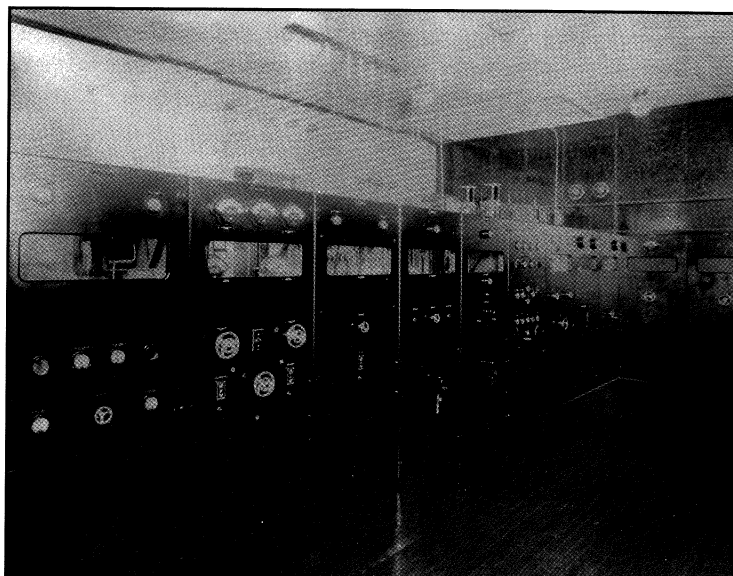
Figure 5. Control panels for the 180-kw station. The modulator tubes in Figure 3 are behind the third and fourth panels from the left, and the power amplifier tubes are behind the eighth and ninth panels. The tank circuit in Figure 4 is on the other side of the wall at the far right in the figure. The plate leads connect to the tank circuit through the feed-through insulators that are visible on the wall.
