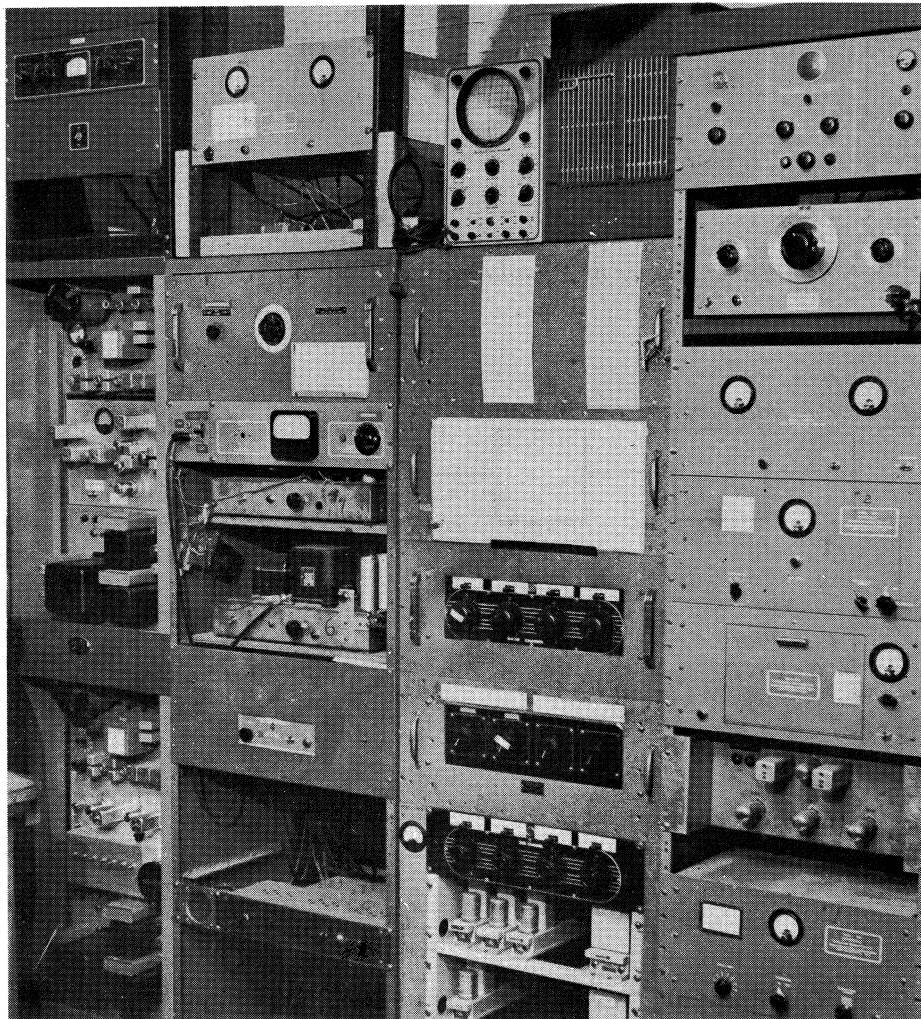
Fig. 5. CONTROL ROOM AT ALPINE -- Main and auxiliary modulation equipment contained in rack on extreme left with Mr. Perry Osborn, Chief Engineer, KE2XCC beside it.
