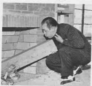
3 The contractor said there'd be a lot of firewood left over. Oh yeah! Eight little pieces and one big hunk which a carpenter later took!
