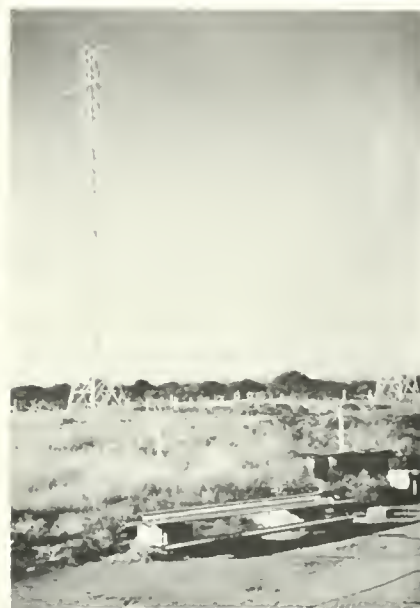
MODERN TOWERS ARE PART OF THE ANTENNA SYSTEM INSTALLED BY THE RADIO CLUB OF MOZAMBIQUE.
