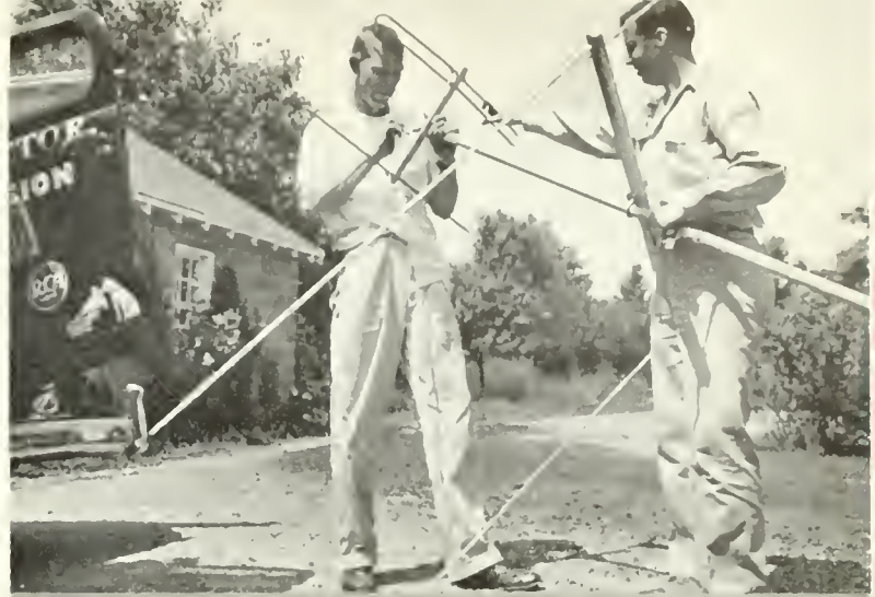
9. A high frequency antenna is added to the main antenna mast to ensure reception of all stations in localities where some signals are weak.
