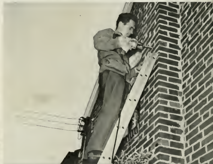
6. Holes are drilled in the side of the house to support hooks for the RCA "Bright-picture" tape which conveys signals to the receiver.
