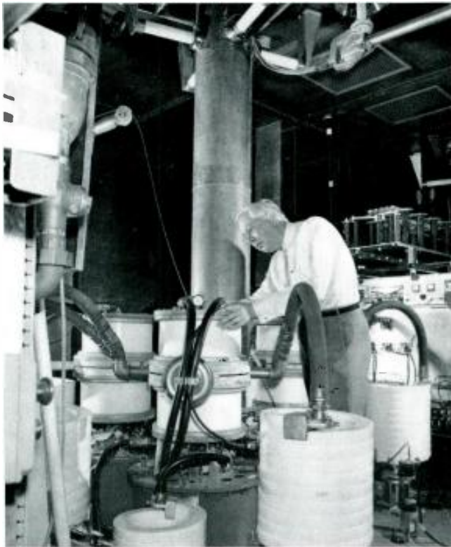
Array of RCA superpower tubes provides heat for C Stellarator.
