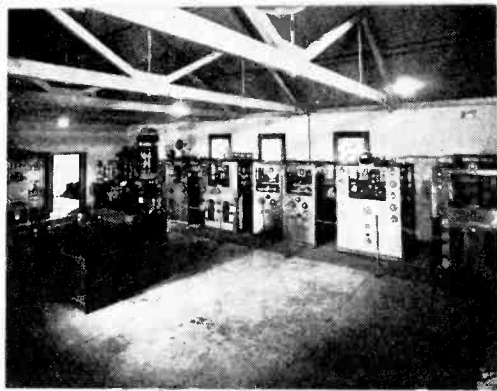
The transmitting studio of VK3ME installed at Braybrook, near Melbourne, Victoria, Australia. This short wave transmitter was designed and manufactured in Australia by Amalgamated Wireless (A'sia) Ltd.
