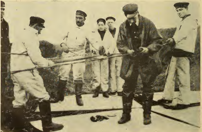
A new telephone cable has been laid between England and Ireland at a cost of $380,000.
