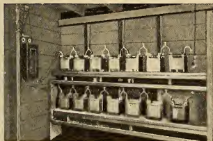
FARM STORAGE BATTERY
