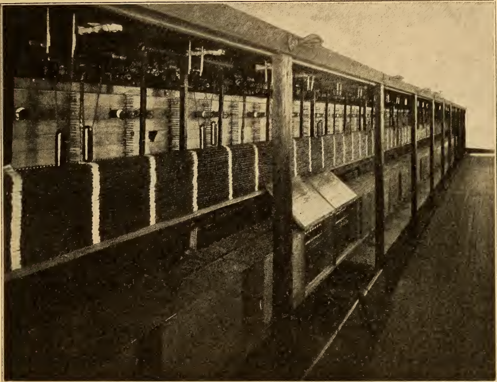
A VIEW OF THE BACK OF A MODERN TELEPHONE SWITCHBOARD. Here are hundreds of miles of wire, tens of thousands of soldered joints.
